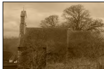
Dilapidated church, no longer in use.
